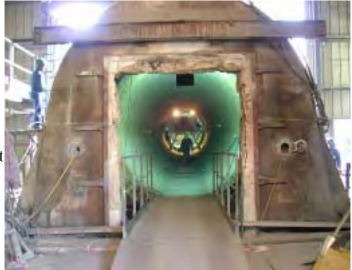
KilnGard™-600SCW Application in a Cement Kiln
