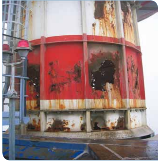
Figure 5. Severely corroded upper section of a stack.
