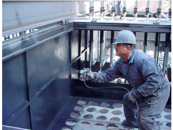
Baghouse Filter Protected with FlueGard-225SQC
